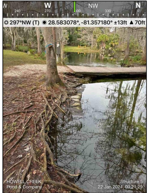
Photograph 14: Structure 5; Subgrade Concrete Bag Retaining Wall (Priority 0)
