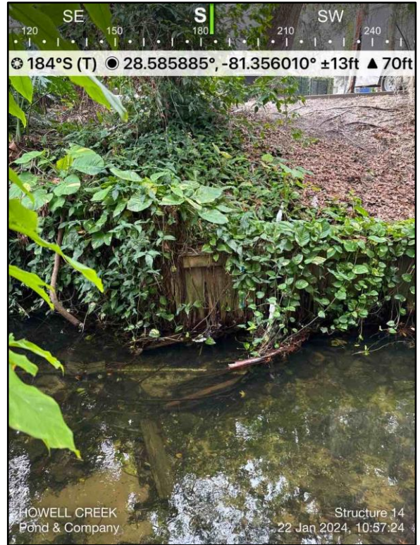
Photograph 34: Structure 14; Wooden/Concrete Bag Retaining Wall at S Penn. Ave. (Priority 4)
