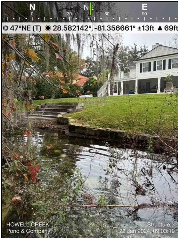
Photograph 7: Structure 3; Block and Mortar Retaining Wall (Priority 2)
