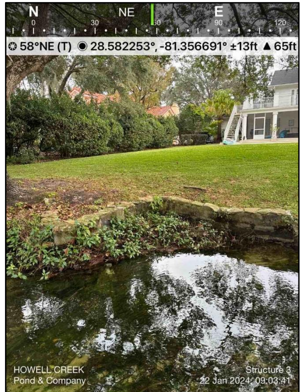
Photograph 8: Structure 3; Block and Mortar Retaining Wall (Priority 2)
