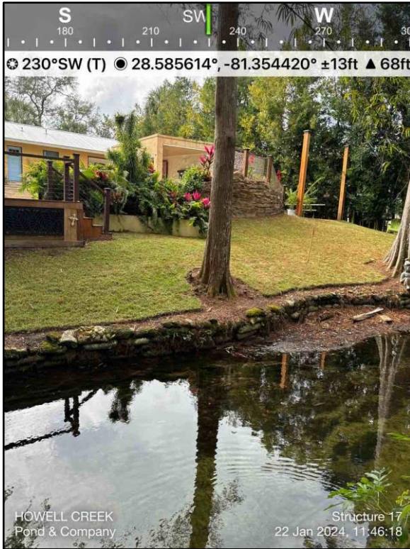
Photograph 41: Structure 17; Concrete Bag Retaining Wall (Priority 0)
