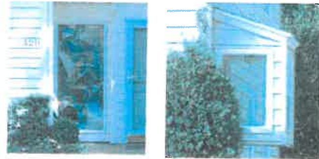
Examples of inappropriate window additions
