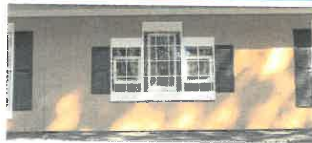
Inappropriate Window Type
