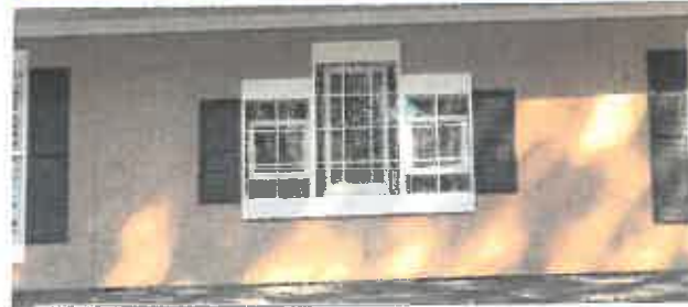
Inappropriate Window Type
