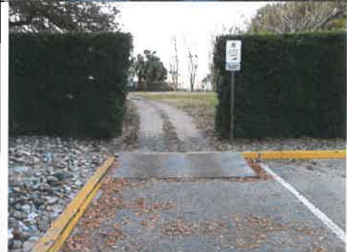
Ramp on parking lot side of Rollins owned commercial property that fronts Fairbanks Ave.
