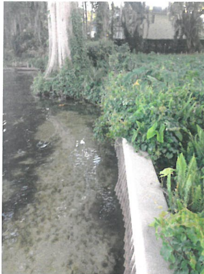
VIEW WEST DAMAGE TO THE SEAWALL PERMITS EROSION TO PORTIONS OF THE SHORELINE
