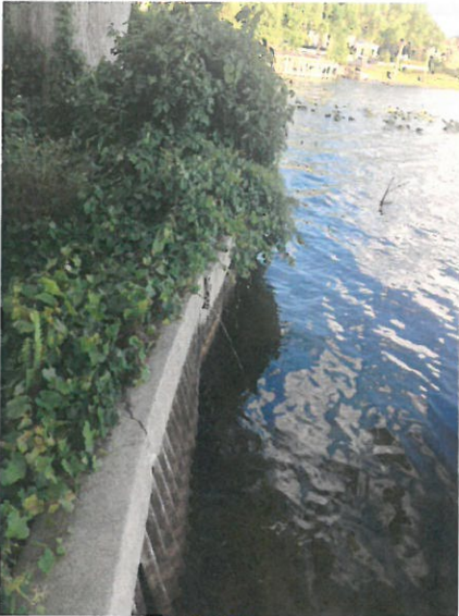
VIEW EAST THE WALL HAS WARPED OVER TIME, CREATING AN UNSIGHTLY AND UNSAFE BULKHEAD.
