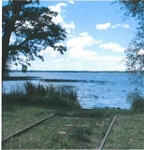
TRACKS INSTALLED WITH LANDSCAPING. THE PRODUCT IS INSTALLED FLUSH ALONG GRADE AND CAN BE PLANTED AND MAINTAINED WITH TRADITIONAL LANDSCAPING.
