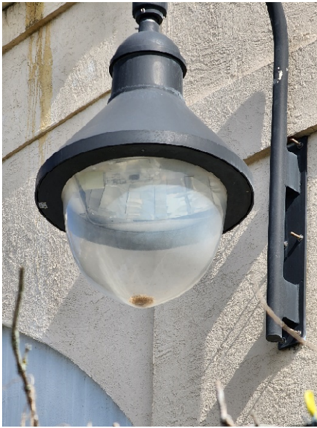
C-5: Exterior Lighting
