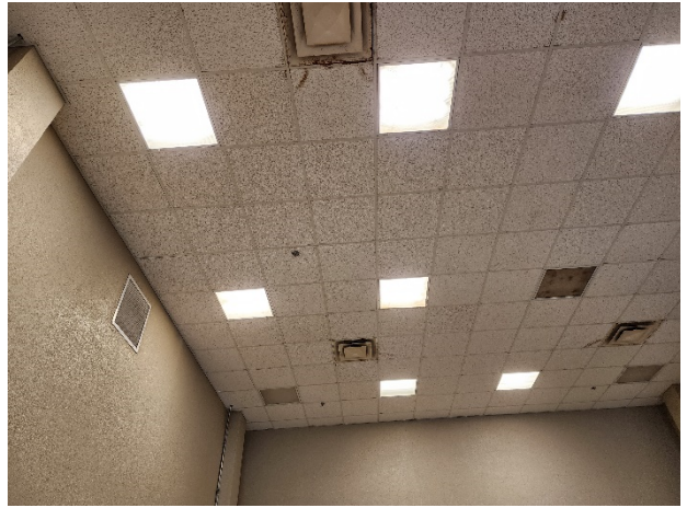
C-8: Interior Lighting
