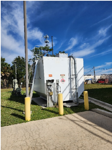
C-3: Exterior Generator Equipment
