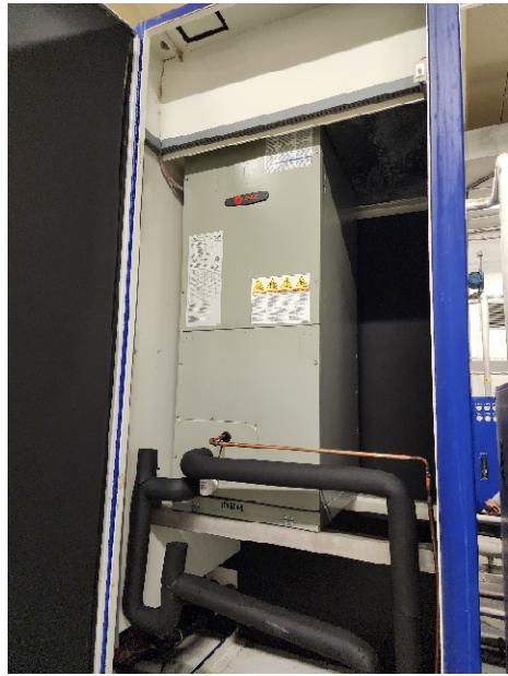
C-18: Trane AHU (2)
