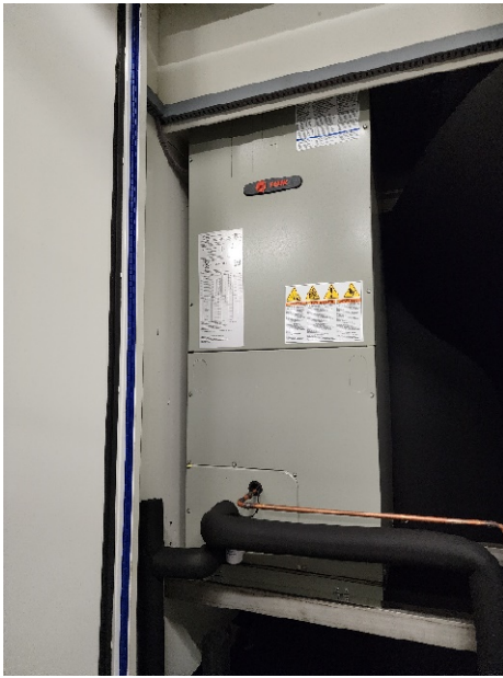
C-17: Trane AHU (1)
