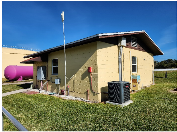
C-6: Condensing Unit (2)
