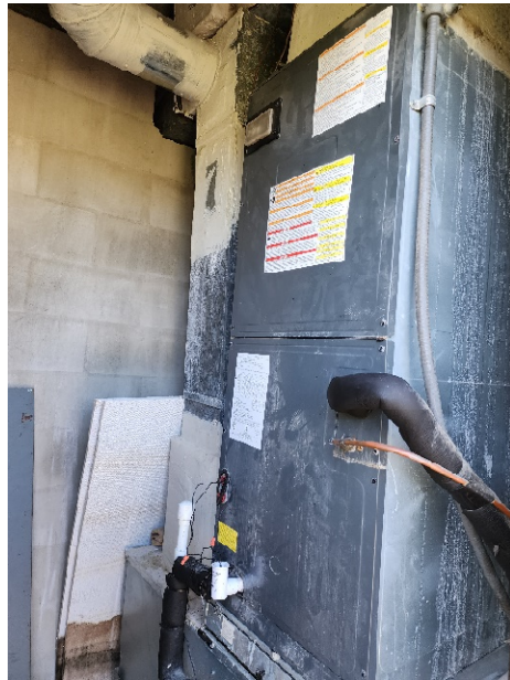
C-4: Air Handling Unit (1)
