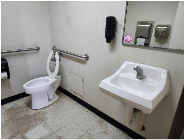
C-5: Restroom Fixtures
