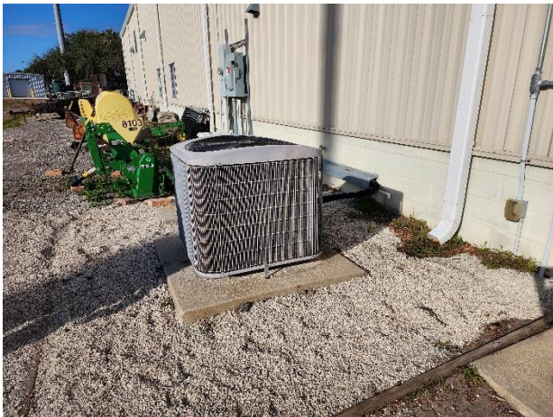
C-7: Condensing Units
