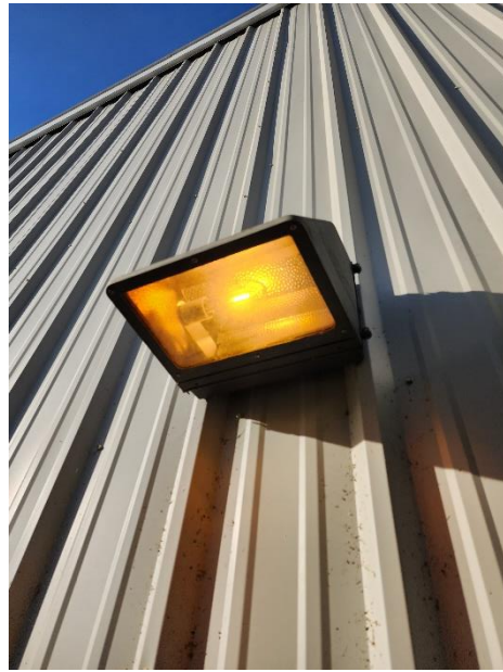
C-6: Exterior Lighting (2)
