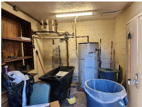
C15: Electric Water Heater
