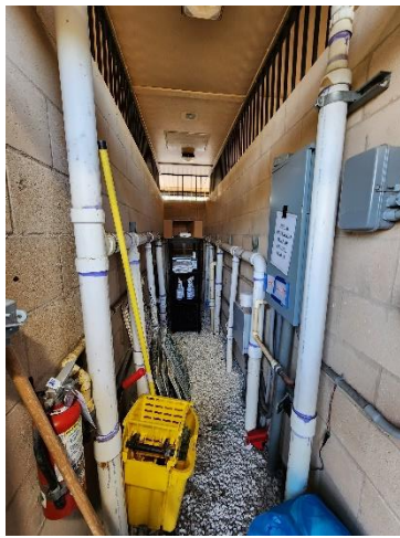
C7: Water Closet
