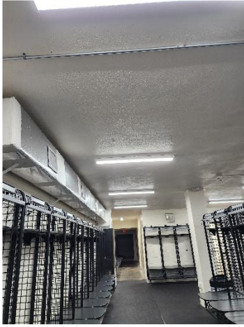
C11: Locker Room Ductwork
