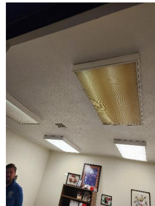
C10: Interior Lighting
