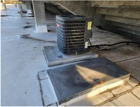
C13: Condensing Unit
