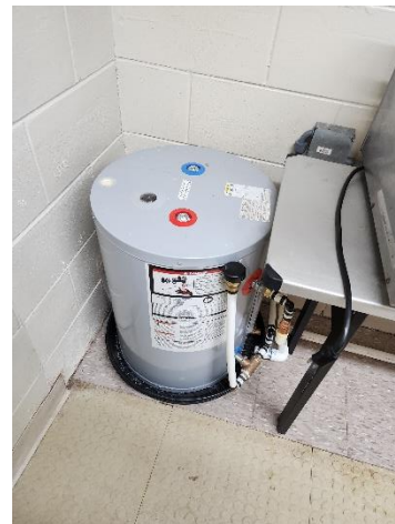
C4: Electric Water Heater
