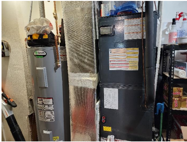
C-5: Water Heater and Goodman AHU
