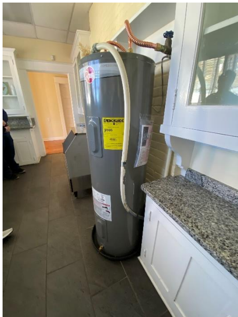
C-11: Clubhouse Electric Water Heater
