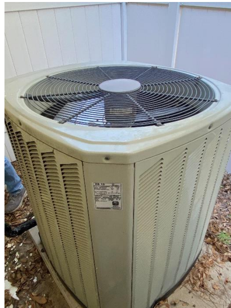
C-8: Clubhouse Condensing Unit (2)
