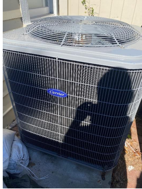
C-6: Pro Shop Condensing Unit
