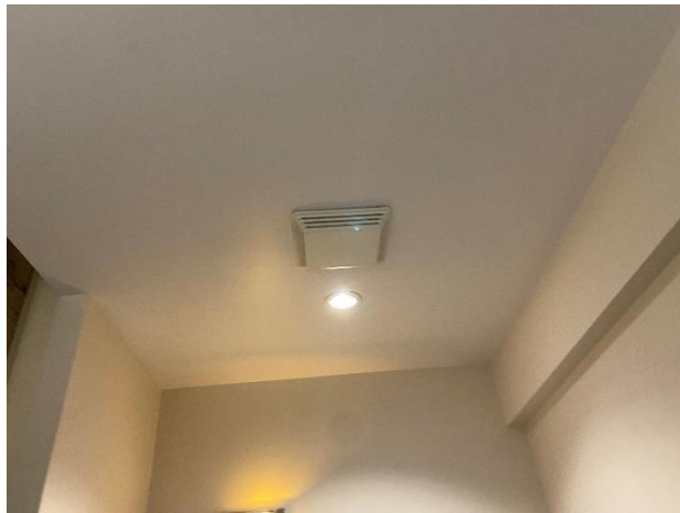
C-3: Pro Shop Bathroom Light and Exhaust Fan
