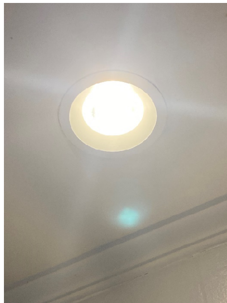
C-4: Kitchen Lighting Fixture
