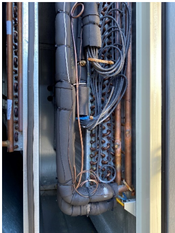
C-7: RTU Cooling Coil (Typical of 3)
