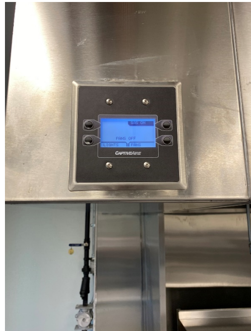
C-16: Kitchen vent hood controls
