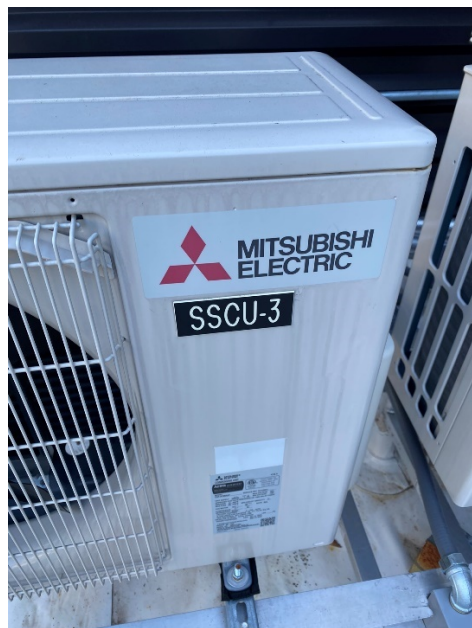
C-12: Split System Condensing Unit SSCU-3
