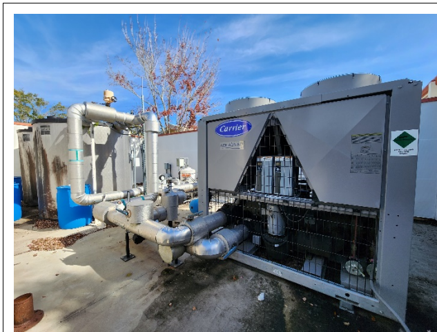
C-1: Air-Cooled Chiller
