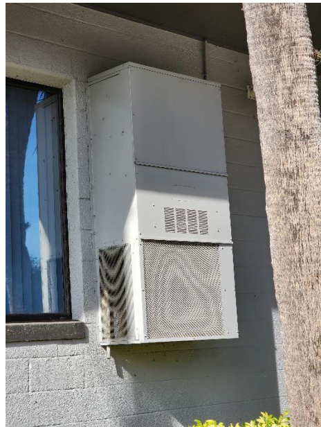
C-4: Packaged Air Conditioning Unit (Photo 1)
