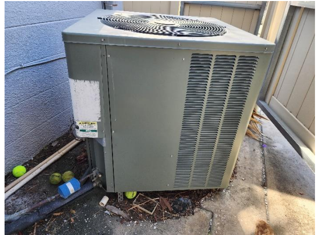
C-2: Condensing Unit (Photo 2)
