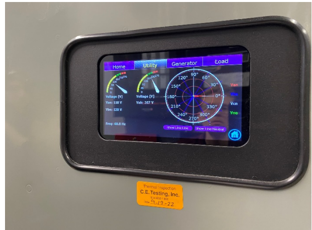
C-24: Transfer Switch Readings
