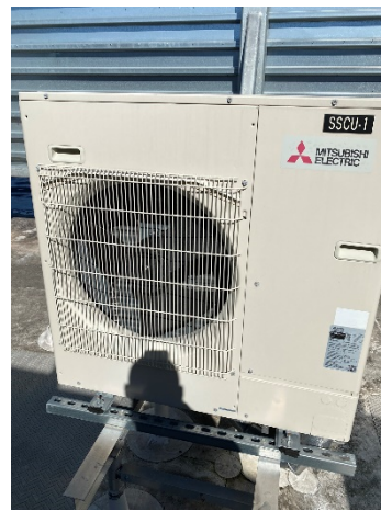
C-12: Split System Condensing Unit SSCU-1
