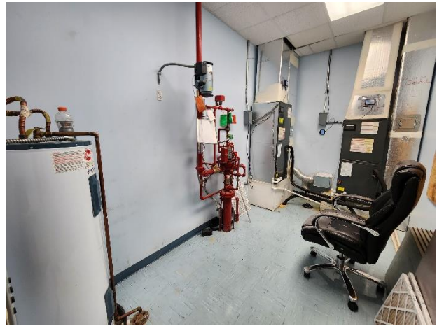
C-10: Electric Water Heater and Air Handling Units
