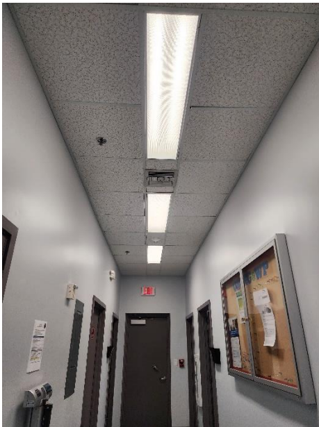
C-7: Hallway fluorescent lighting
