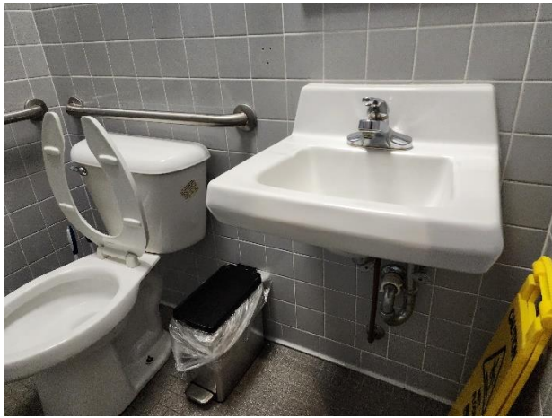
C-5: Restroom fixtures
