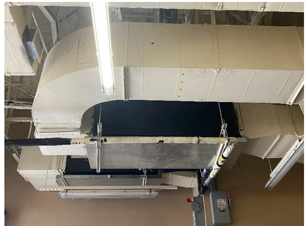
C-8: Air Handling Units
