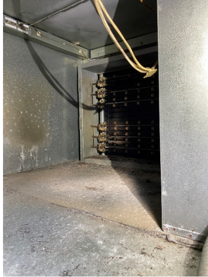
C-21: AHU-4 Heating Coil Condition
