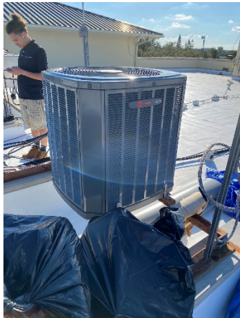
C-8: Trane Rooftop Condensing Unit
