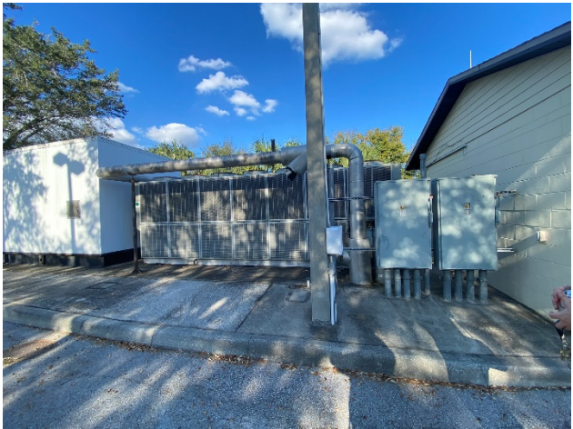
C-12: Air-Cooled Chiller CH-1
