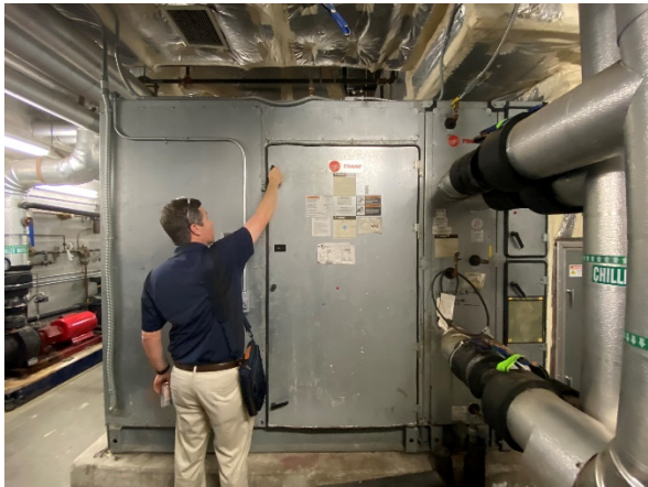
C-15: Air Handling Unit AHU-1
