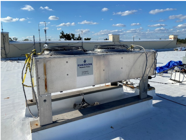
C-7: Emerson CRAC Condensing Unit
