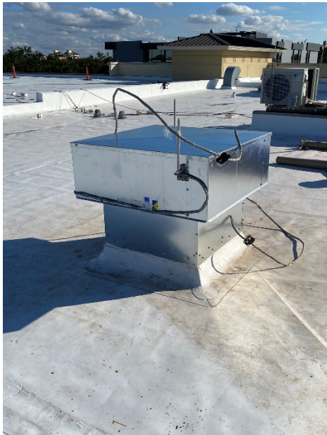
C-10: Rooftop Outside Air Fan
