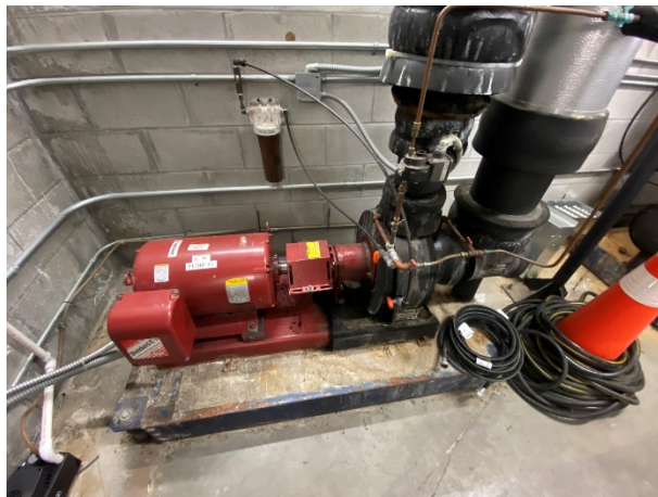
C-17: Chilled Water Pump
