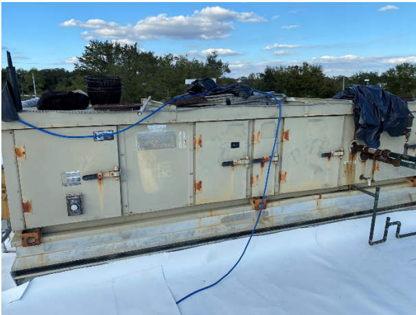
C-19: Air Handling Unit AHU-4
