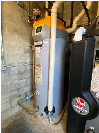
C-23: Gas-Fired Water Heater (2)
