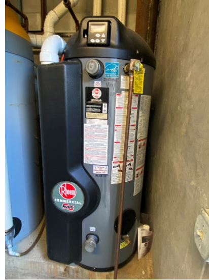
C-22: Gas-Fired Water Heater (1)
