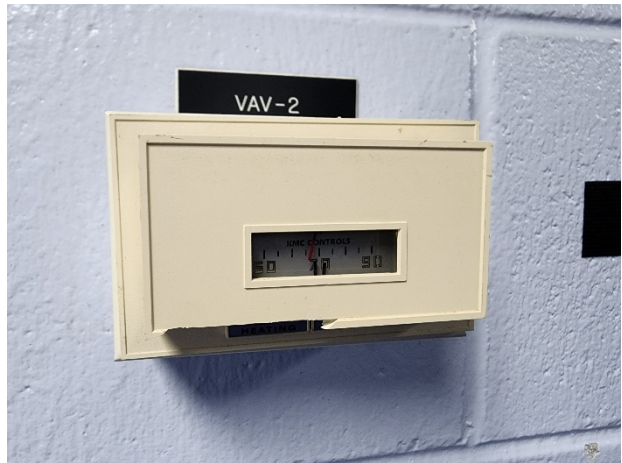
C-8: VAV-2 Controls
