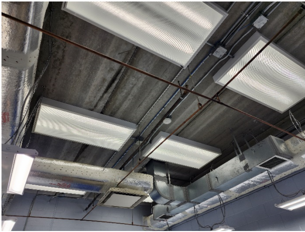
C-13: Interior Lighting
