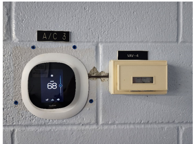
C-10: A/C-3 Thermostat and VAV-4 Controls
