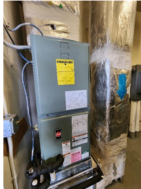
C-8: Air Handler
