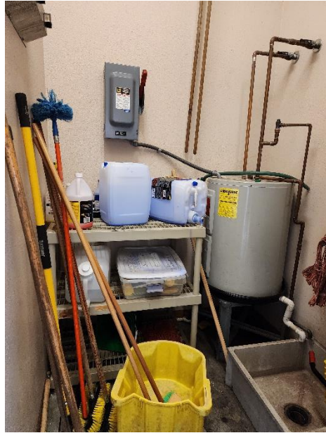
C-9: 40 Gallon Electric Water Heater
