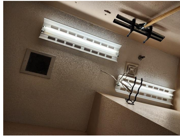
C-10: Station Lighting
