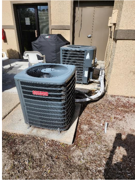
C-7: Condensing Units
