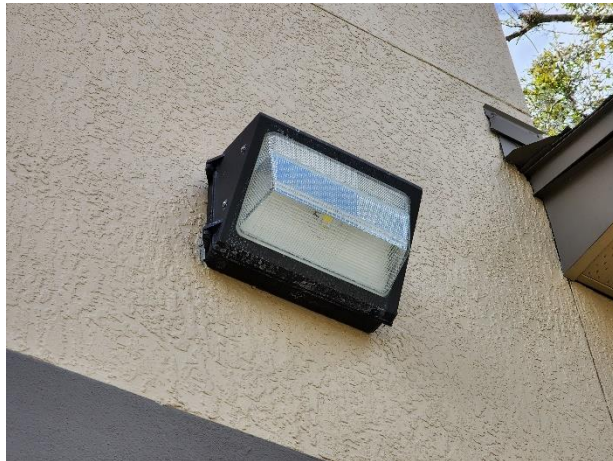
C-15: Exterior Lighting
