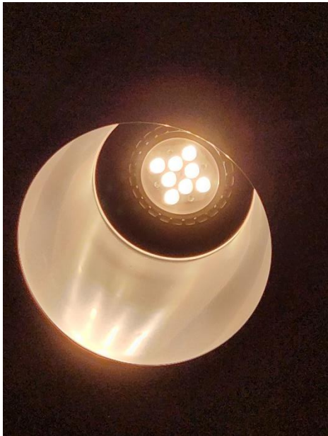
C-4: Fire Station lighting
