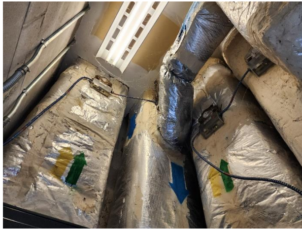
C-13: Air Handler ducts
