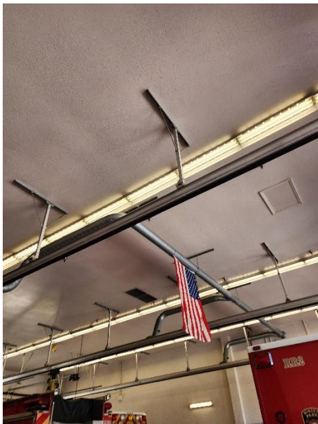
C-2: Garage lighting
