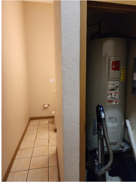
C-5: 86 Gallon Electric Water Heater
