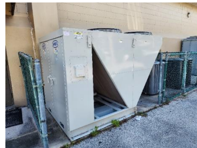
C18: Air Cooled Chiller
