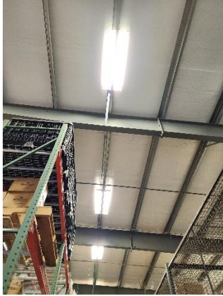
C35: Interior Lighting
