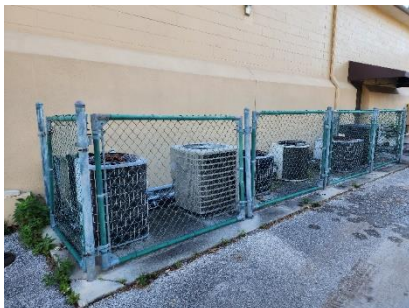
C17: Condensing Units
