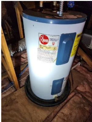
C15: Electric Water Heater
