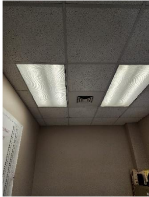
C26: Interior Lighting
