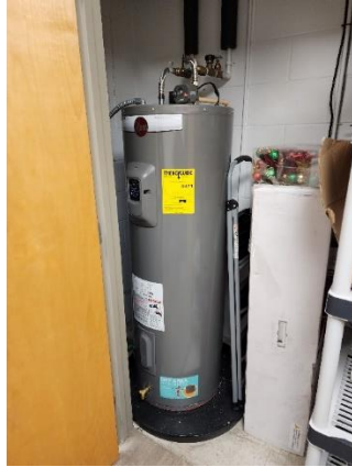
C5: Electric Water Heater
