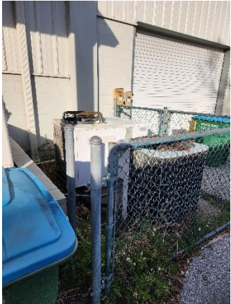
C25: Condensing Units
