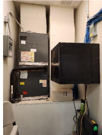
C36: Air Handling Unit
