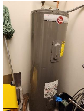
C34: Electric Water Heater
