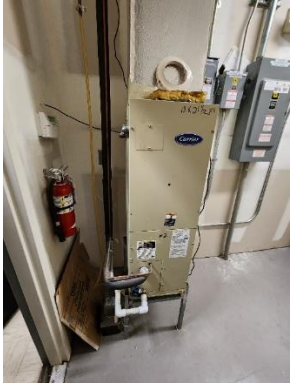
C23: Air Handling Unit
