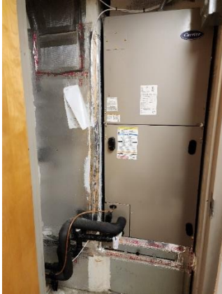
C3: Air Handling Unit
