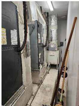
C28: Air Handling Units
