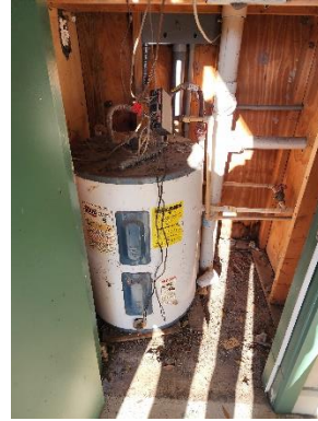
C31: Electric Water Heater
