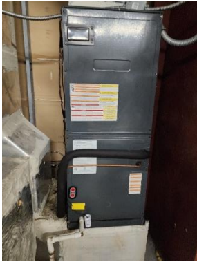
C24: Air Handling Unit
