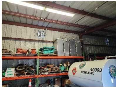
C32: Interior Lighting and Ventilation Exhaust Fan
