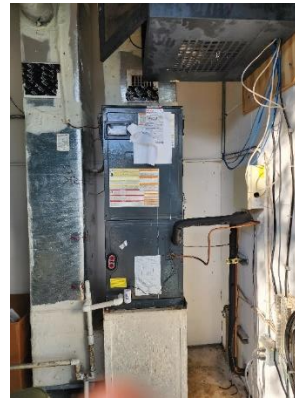
C16: Air Handling Unit
