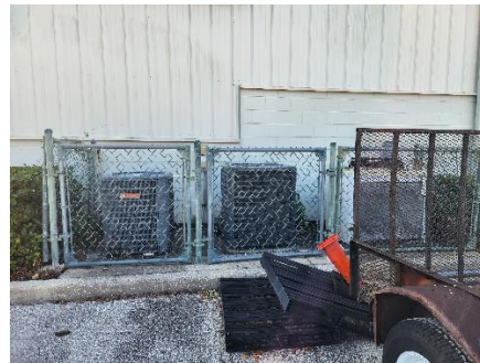
C29: Condensing Units
