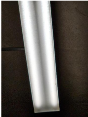
C37: Interior Lighting
