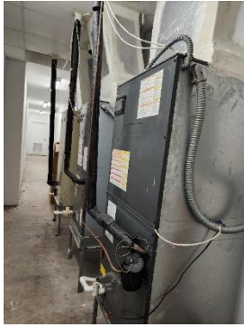
C19: Air Handling Units
