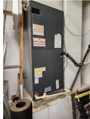
C6: Air Handling Unit
