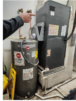
C27: Electric Water Heater and Air Handling Unit
