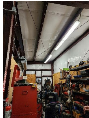
C38: Storage Exhaust Fan
