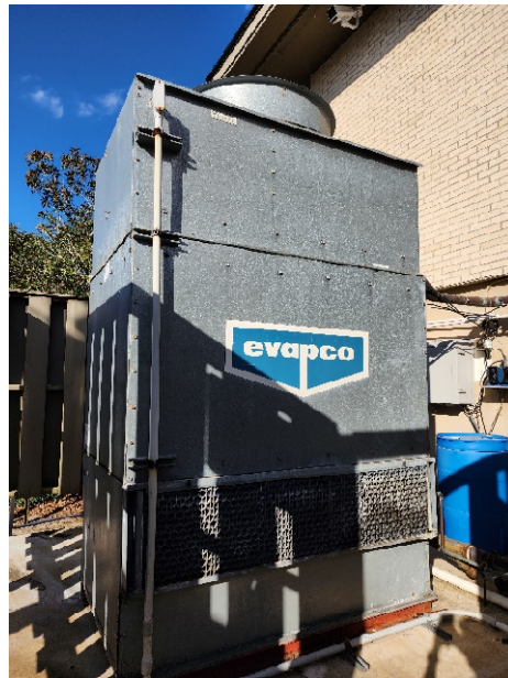
C-24: Cooling tower
