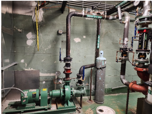
C-11: Condenser water pump
