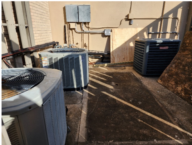
C-23: Condensing units
