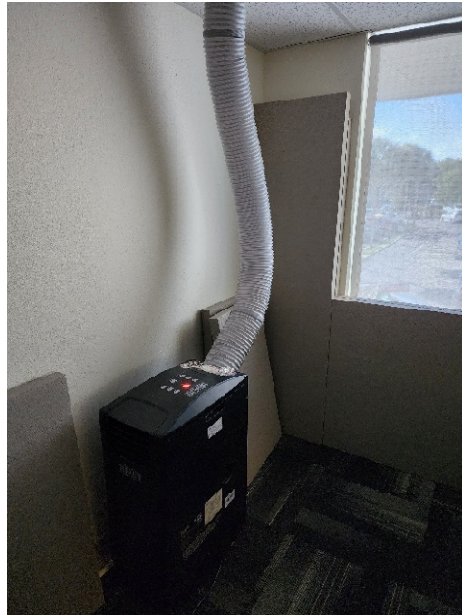
C-14: Portable AHU
