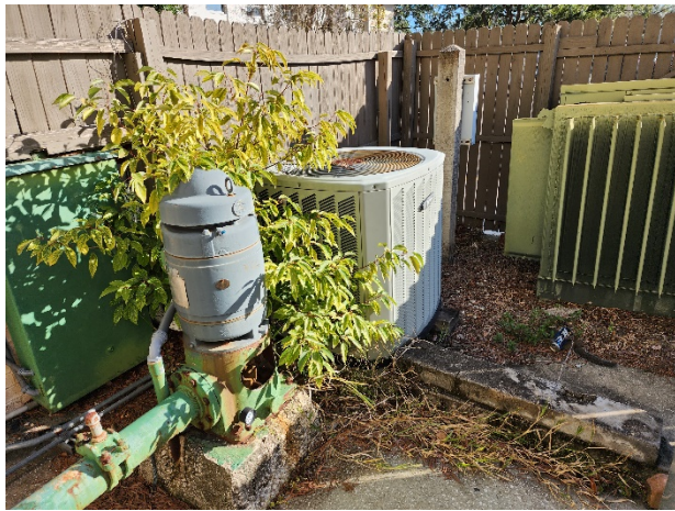
C-21: Trane condensing unit
