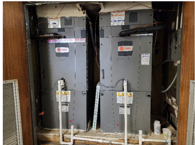
C-16: Air handling units
