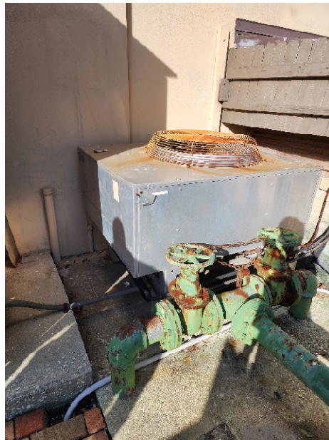
C-22: Liebert condensing unit
