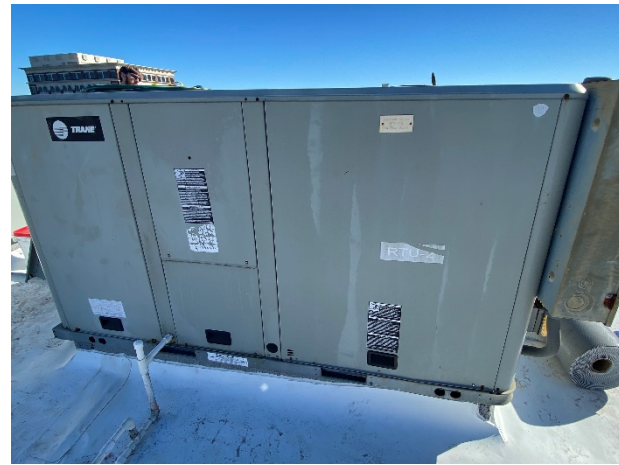
C-4: Packaged RTU (photo 2)
