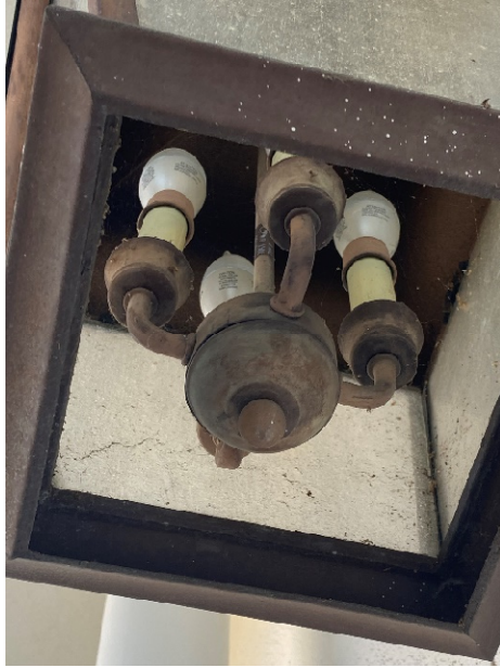
C-11: Exterior Lighting Fixture
