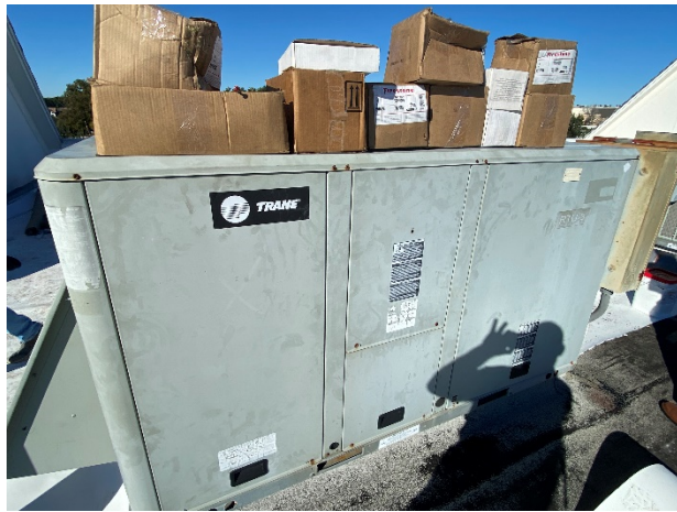
C-5: Packaged RTU (photo 3)
