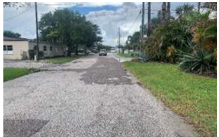
Observed examples of defective or inadequate street layout, roadways, and parking facilities within the Fairbanks Avenue FON Study Area.
