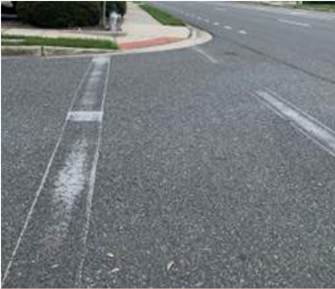
Deteriorated cross-walk markings.
