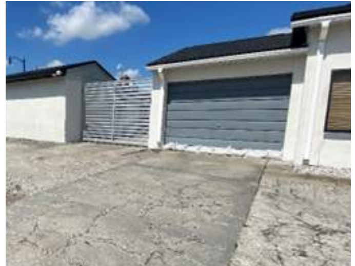
Deteriorated signage and parking improvements.
