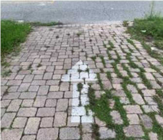
Deteriorated brick driveway.
