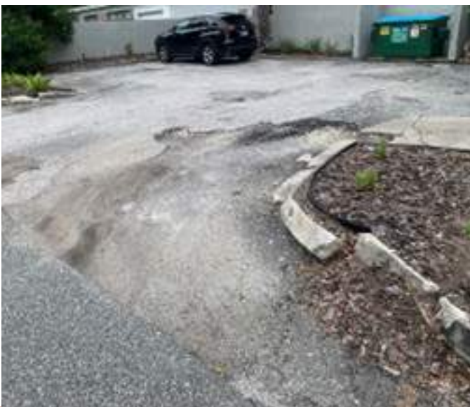
Deteriorated parking lot entry apron and curb.
