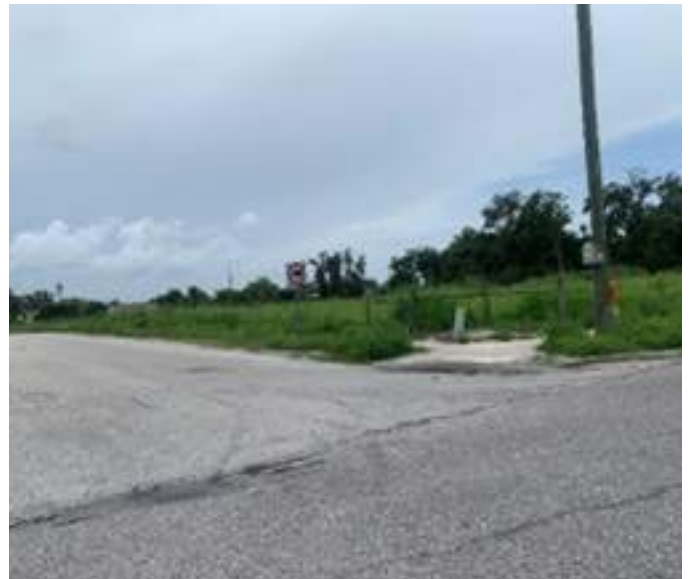
Defective street layout. Sidewalks and roadway serving large undeveloped, superblock, parcels near Rauvadage.
